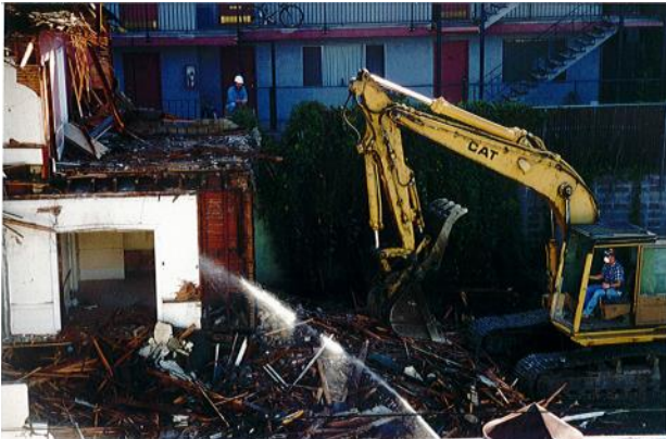
In June the bulldozers demolish the apartment building on Montecito to make way for a playground.
